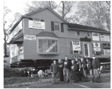
Recently, the Levi Cory House was moved to a new location on Constitution Plaza. Members of the Mountainside Restoration Committee pose before the house where it currently is suspended upon cribbing.
