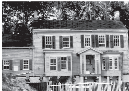
In the summer of 1985, the Deacon Andrew Hetfield House sat atop cribbing on Constitution Plaza waiting for its foundation to be poured before it was lowered onto a new basement and foundation.
